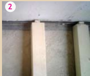
2 FIX OF THE IPE 120 AND OF THE JOISTS TO THE MAIN WALLS
