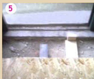
5 FIXING OF THE IPE BEAM AND OF THE JOISTS CLOSE TO THE THRESHOLD OF BALCONY
